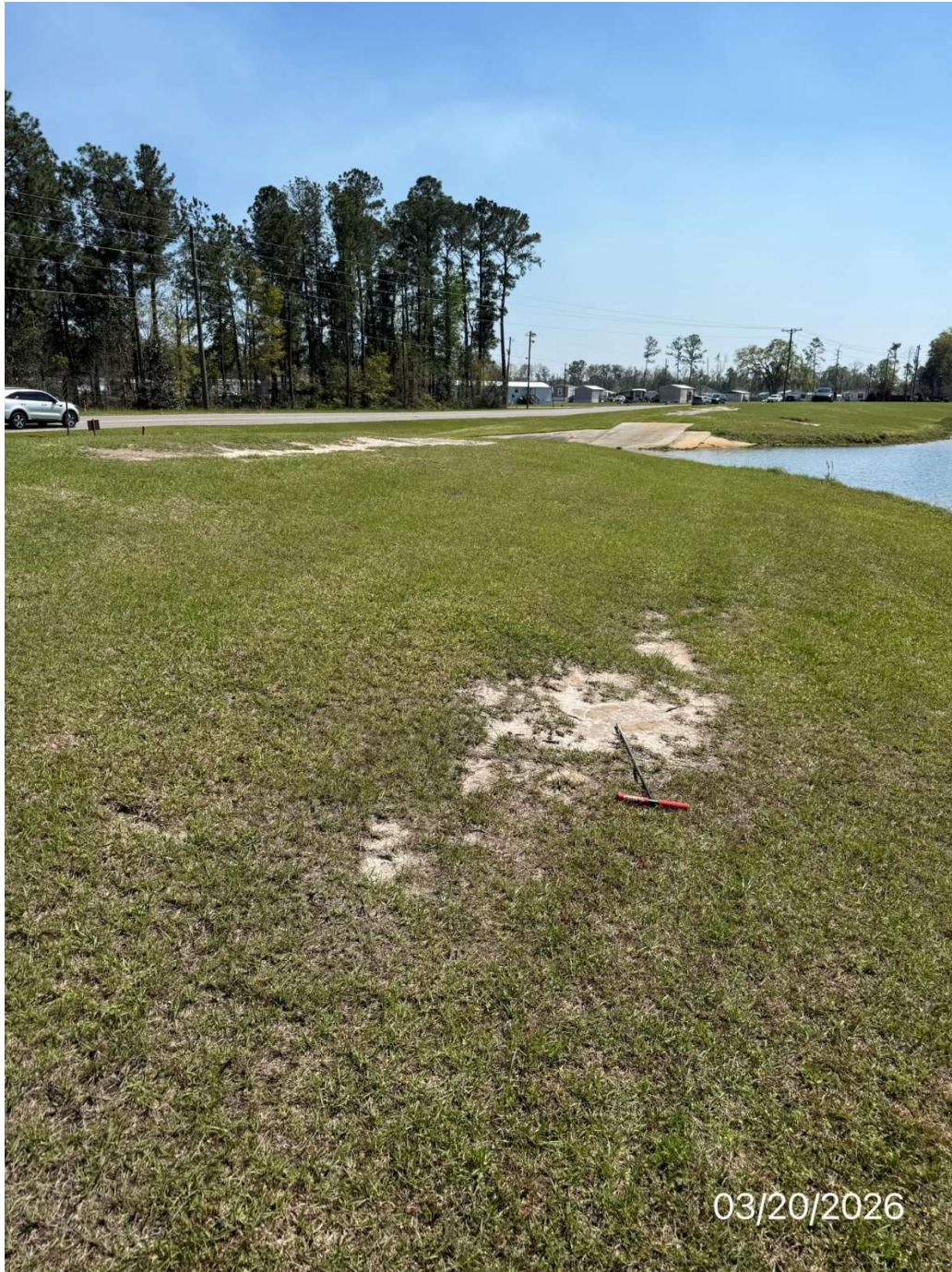
Picture #6 - Upstream slope located north of the principal spillway. Add soil to replace eroded bare spots and grass. ( \pm 20 \times 6' area)
