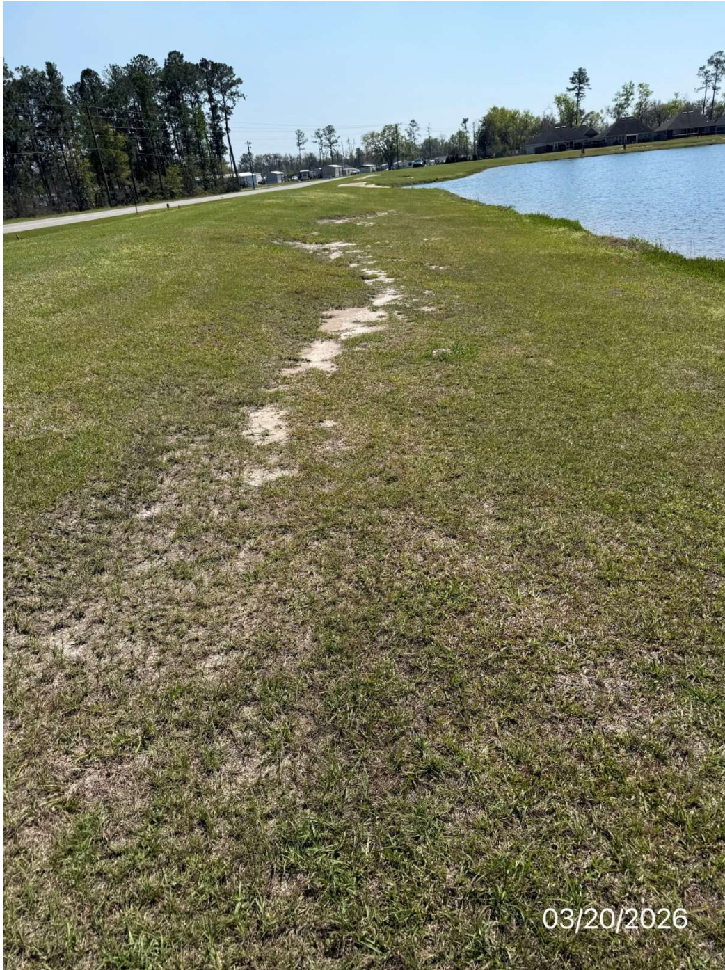
Picture #5 - Upstream slope located north of the principal spillway. Add soil to replace eroded bare spots and grass (+120 x 15' area)
