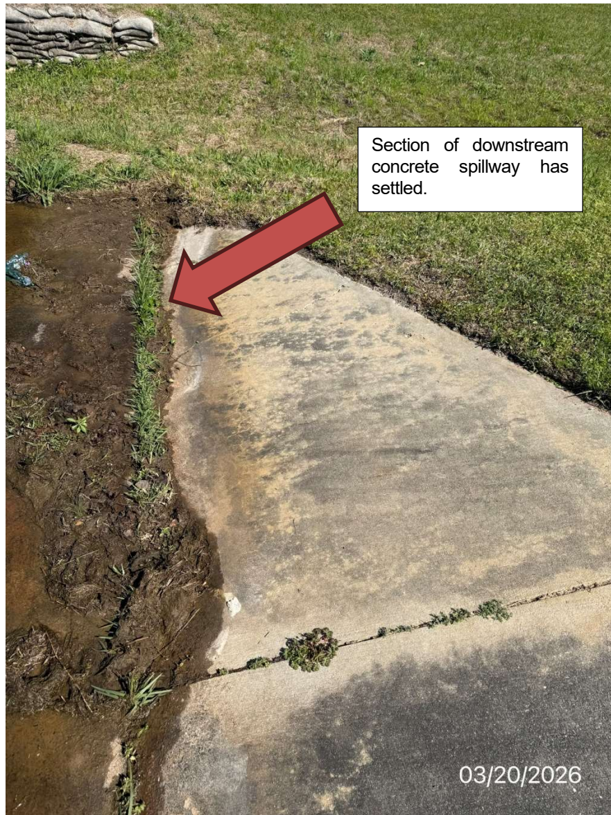
Picture #11 - Concrete slab at the southeastern corner of the concrete spillway. Downstream slope, slight settlement.
