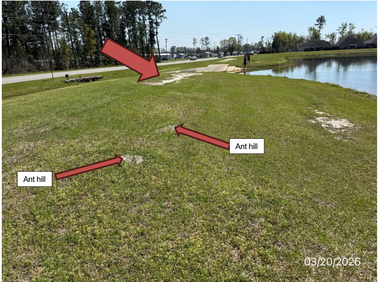
Picture #3 - Crest Condition north of the concrete spillway. Add soil and grass ( \pm 40' \times 10' ) Multiple ant hills need to be removed over length of dam.
