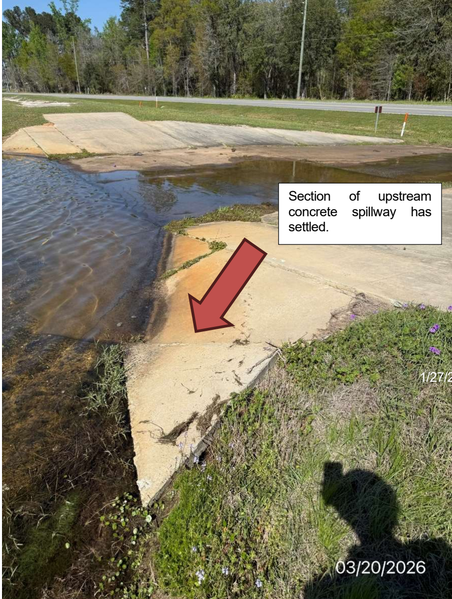
Picture #12 - Concrete slab at the southwestern corner of the concrete spillway. Upstream slope, slight settlement.
