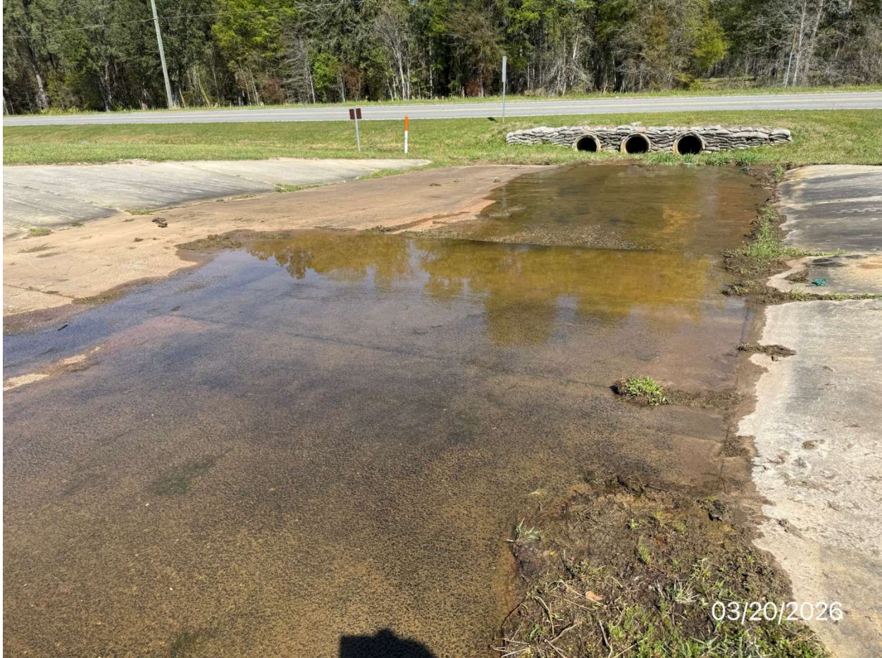
Picture #10 - Principal Concrete Spillway Channel. (Triple 30" RCP culverts under Val Der Road are shown in the background. These culverts are not a part of the dam or outlet system)
