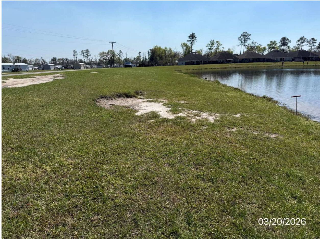
Picture #7 - Upstream slope located south of the principal spillway. Add soil to replace eroded bare spots and grass. ( \pm 20 \times 15' area, about 10" to 12" required)
